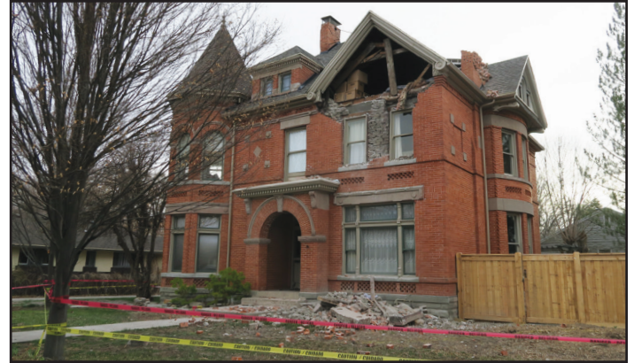
Structural damage from ground shaking to the historical Sears Mansion in Salt Lake City. This home was subsequently demolished due to the extensive damage. Photo courtesy of the Utah Geological Survey.
