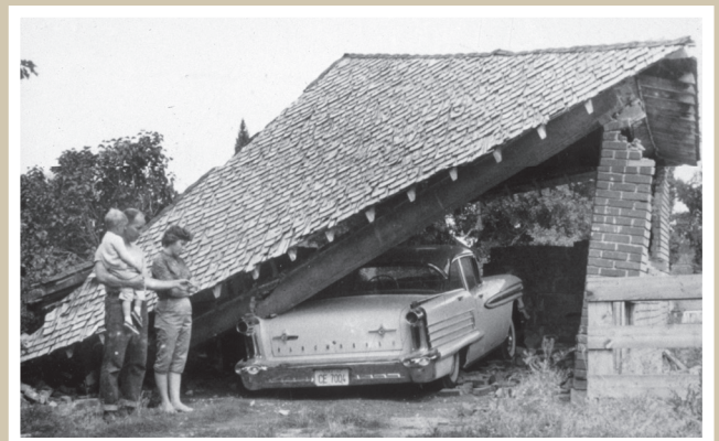
Ground shaking from the 1962 M 5.8 Richmond earthquake caused this brick garage to collapse onto a car. Photo courtesy of The Ogden Standard Examiner.
