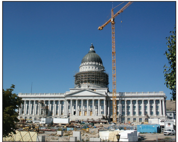
The State of Utah renovated the Capitol Building to preserve a historic building and to ensure public safety and continuity of government in the event of a large earthquake. The Capitol Building rests on a system of 265 seismic base isolators, separating the building from the foundation and lessening the effects of earthquake shaking. Photo taken September 24, 2006, courtesy of the Utah Geological Survey.
