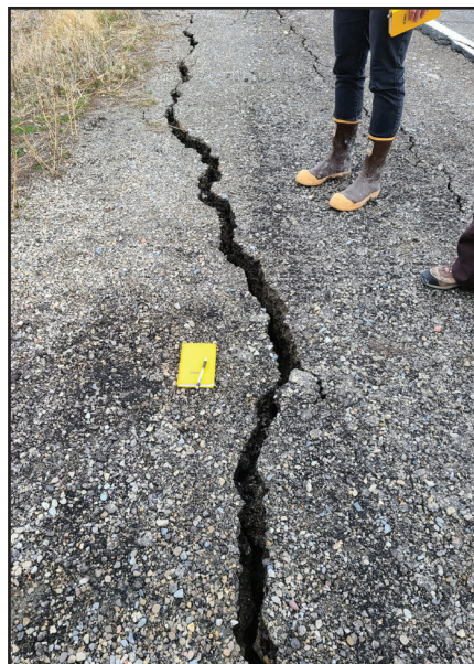
Lateral-spread ground cracking along the Great Salt Lake Marina access road from the Magna earthquake. Photo courtesy of the Utah Geological Survey.
