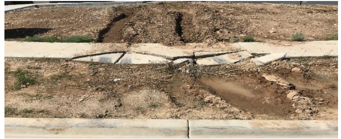
Drive heavy vehicles or equipment over unprotected concrete
